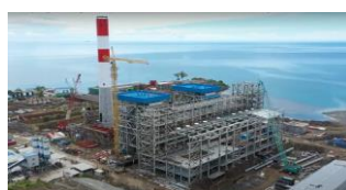
GLP Main plant
