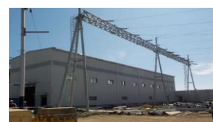
GLP 150 kV GIS Room
